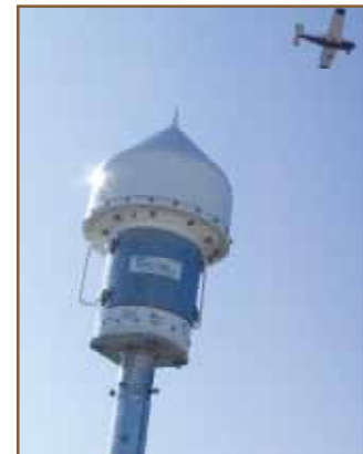
Wide Area Augmentation System (WAAS) GPS Ground Reference Station Antenna
